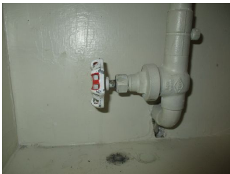
This is the all water shutoff
