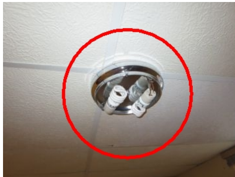
Missing light fixture in basement
