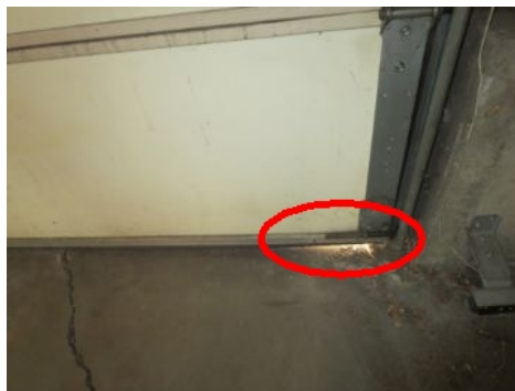
Gap beneath garage door weatherstripping
