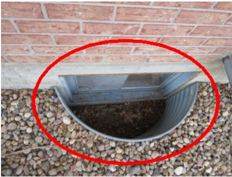
Missing window well covers
