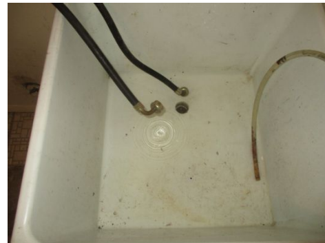
Slow drain at basement laundry sink
