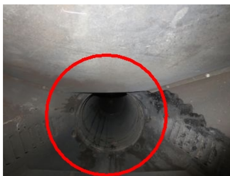
Missing damper in fireplace
