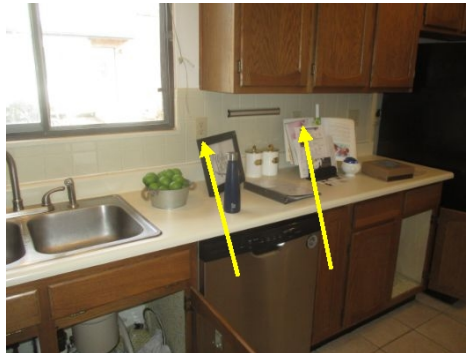
GFCI protection needed in kitchen
