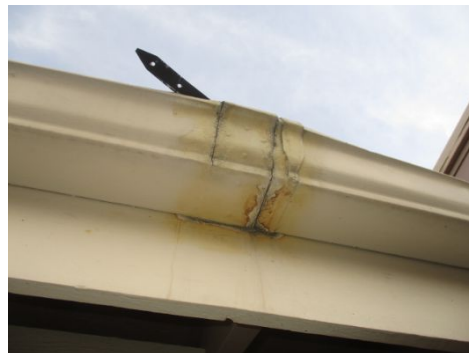
Evidence of previous leaking
