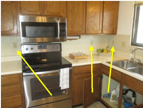
GFCI protection needed in kitchen
