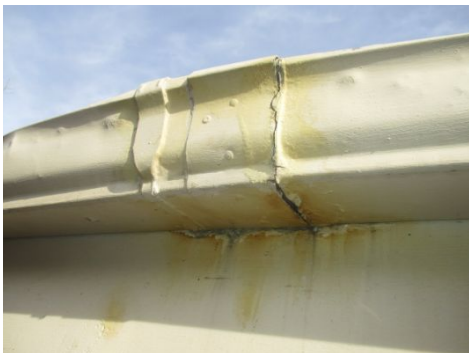
Evidence of previous leaking
