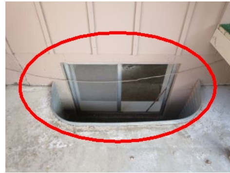
Missing window well cover
