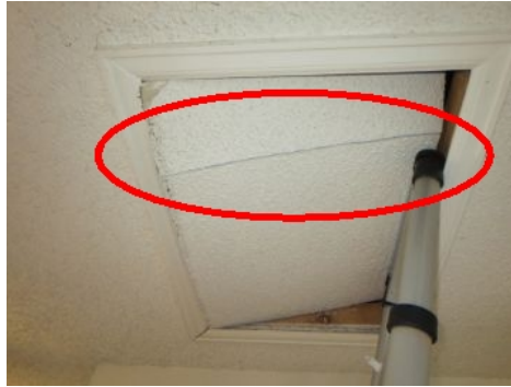
Damaged scuttle hatch
