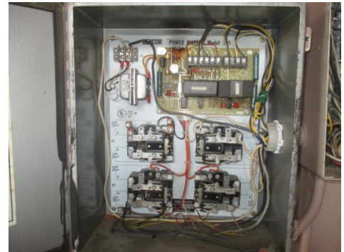
Dencor junction box
