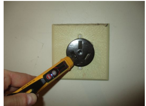
No power detected at basement laundry outlet
