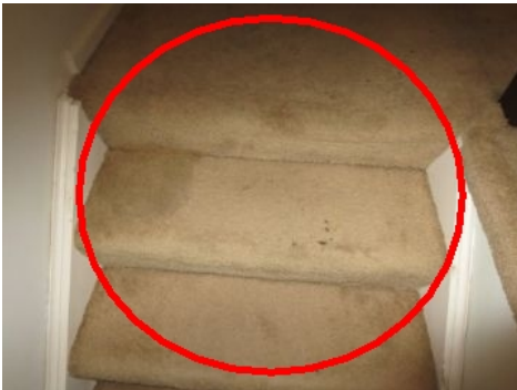
Multiple stains throughout carpeting
