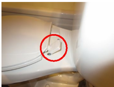
Damaged toilet lid bracket in 2nd floor bathroom
