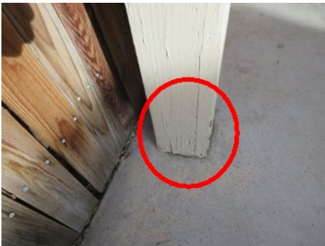
Peeling paint along rear deck support
