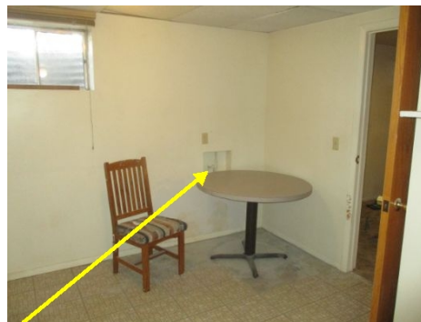
All water shutoff located at front basement wall in laundry room
