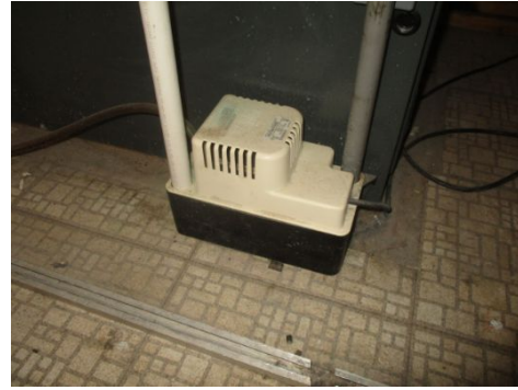
This is the condensate pump
