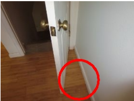
Missing door stoppers throughout home
