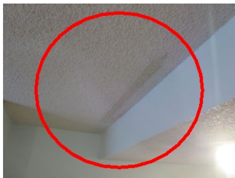
Apparent moisture staining above the living room
