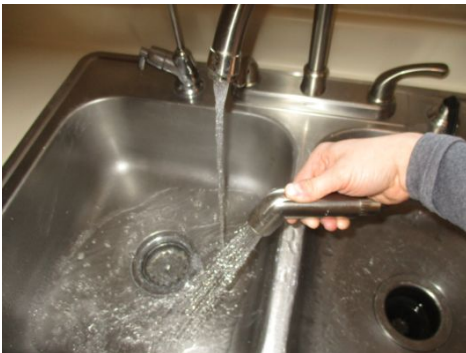
Defective diverter valve
