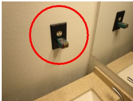
No GFCI outlets located in bathrooms or garage
