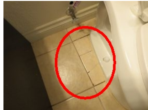
Cracked tiles along the 1st floor half bathroom
