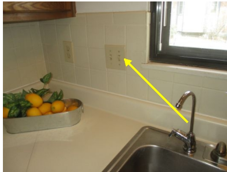
Reverse function at this kitchen sink switch
