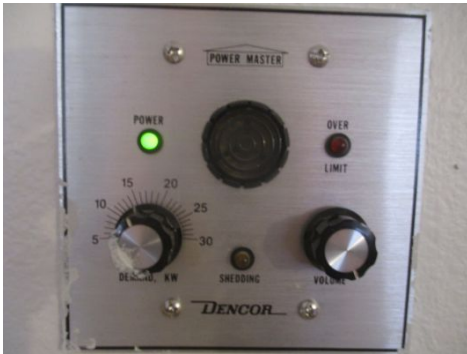
Control panel in living room
