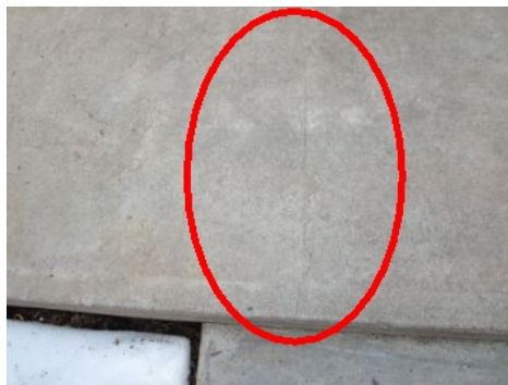
Curing fissure along front porch
