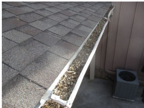
Gutters require cleaning
