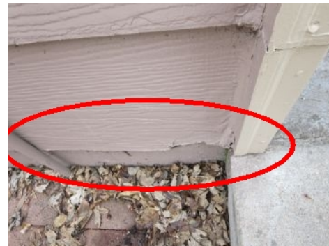
Minor wood rot along garage siding
