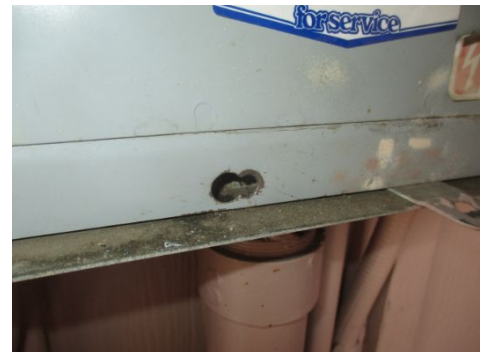
Panel cover screw could not be secured
