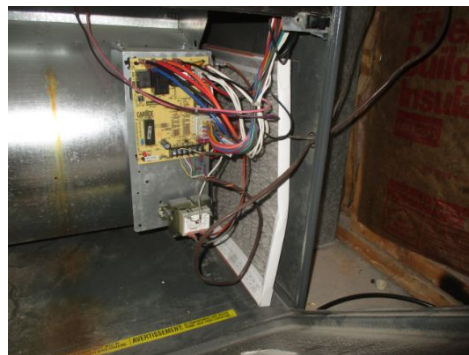
Filter loosely installed
